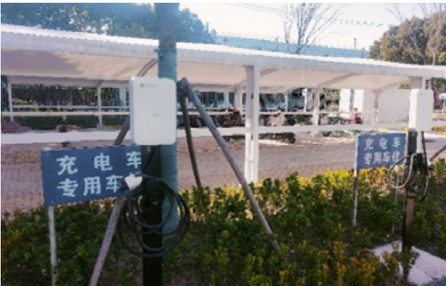
Electric vehicle charging stations
