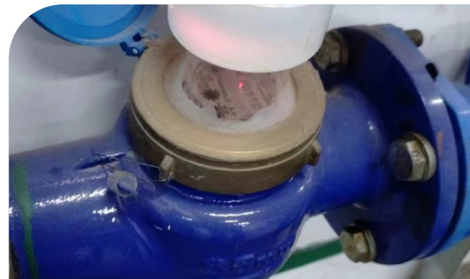
AMR system and smart meters in our logistics industrial distribution warehouses
