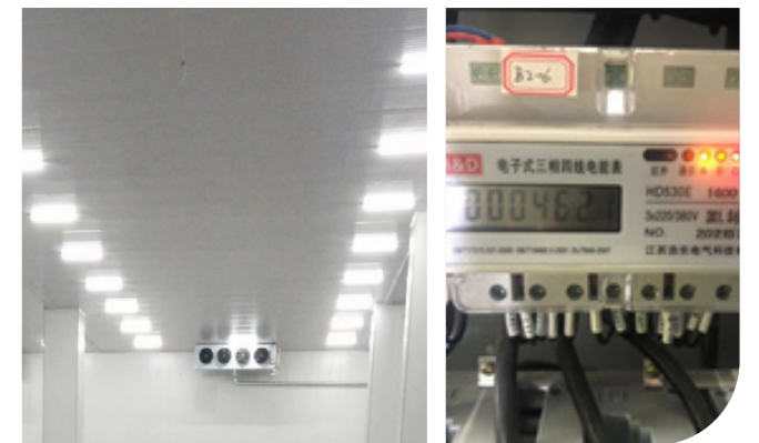
LED lighting system in the logistic industrial distribution warehouses
