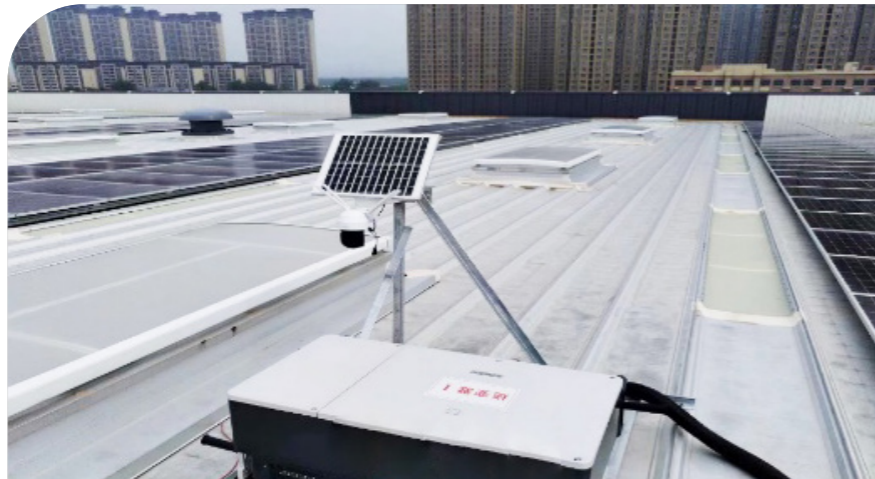
Solar photovoltaic system in Forest Xi'an ETDZ Logistics Park
