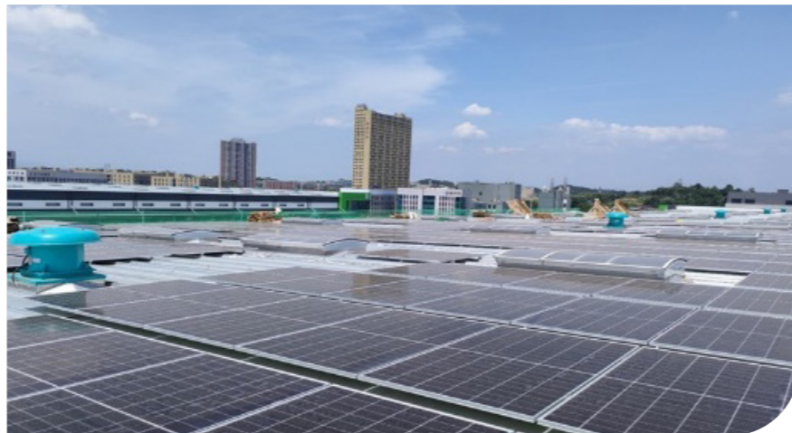
Solar photovoltaic system in Forest Changsha Jinxia Logistics Park
