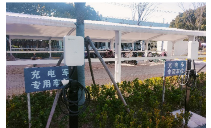
Electric vehicle charging stations
